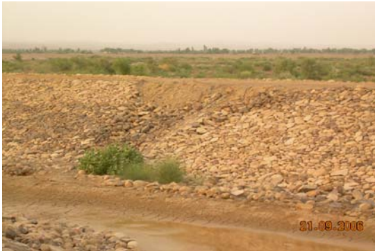
Collapsed slope protection due to undermining
